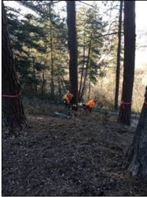
One of the work sites. This cluster of pines was in poor health, leaning uphill towards a homeowner's house, in an area with constant winds and no windbreak.
