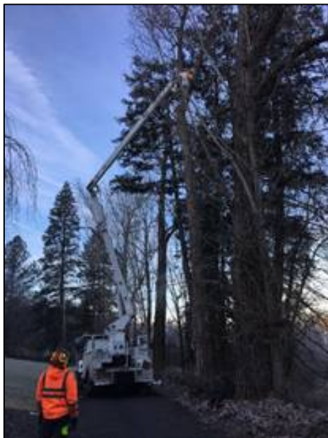
State Parks had to get the bucket truck for some of the trees that had an unfavorable lean.
