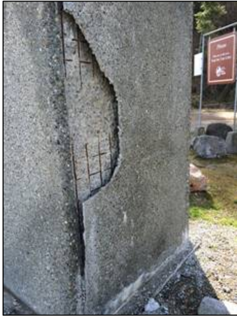
Failing concrete at Loon Lake
