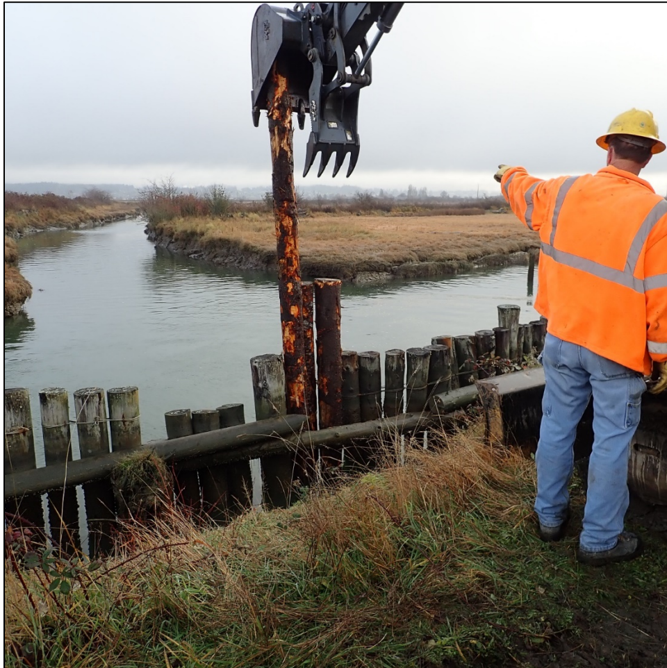
A WDFW construction crew completed the first phase of construction, which involved repairing a wood wall that protects against erosion on a neighboring property
