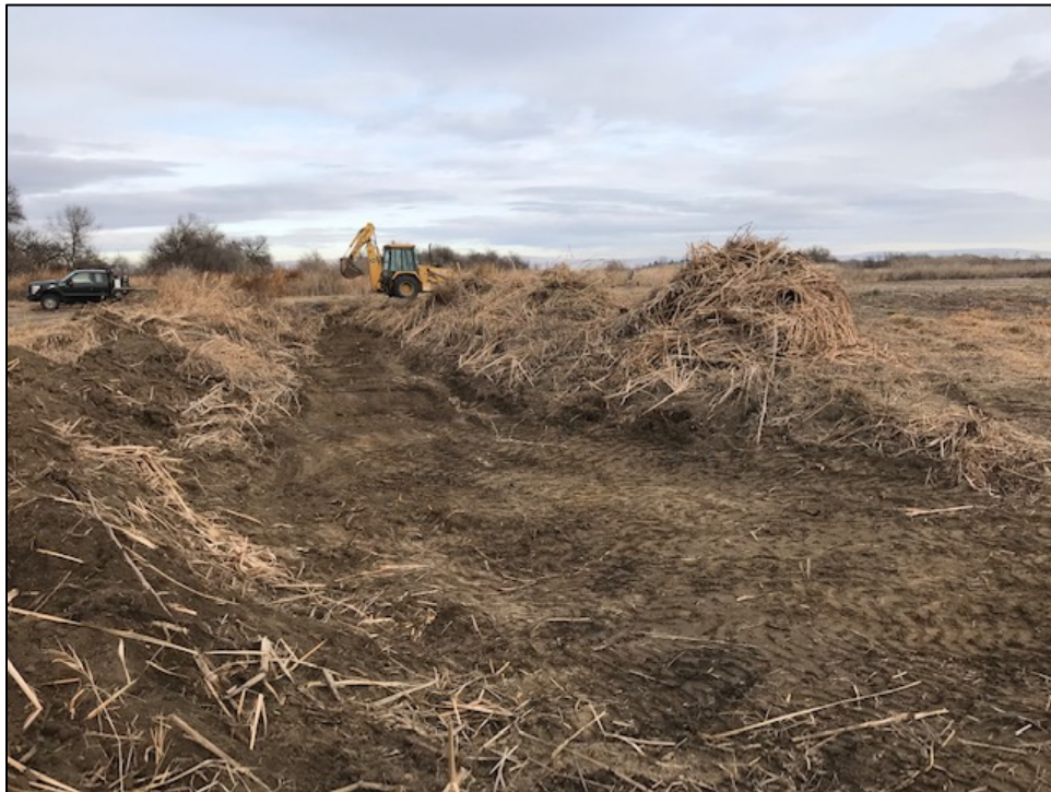
Cattails cleared out of path of water flow, downstream of old culvert structure
