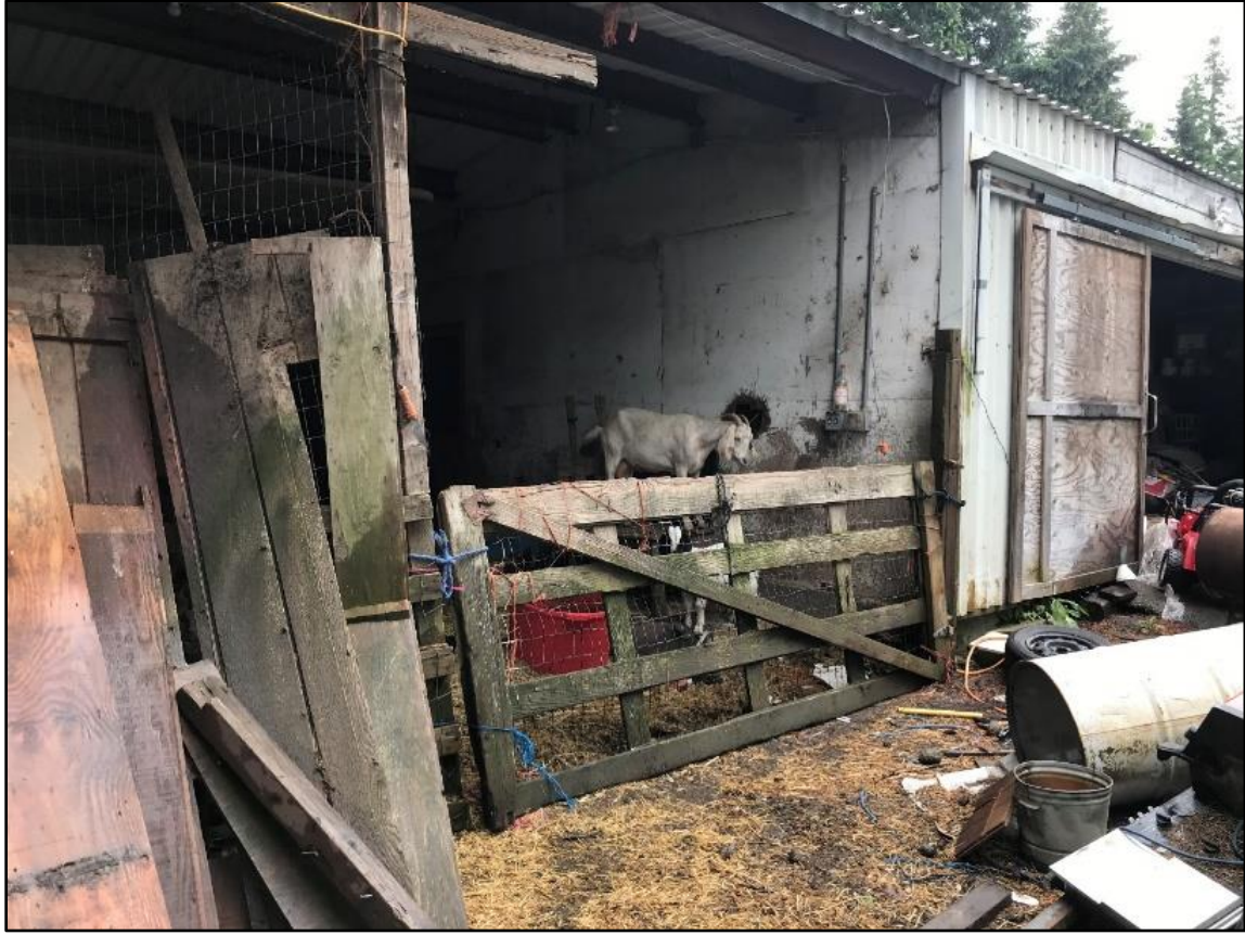
Remaining goats in an unsecured structure, advice was given on reinforcing the goat pen to protect them from wildlife
