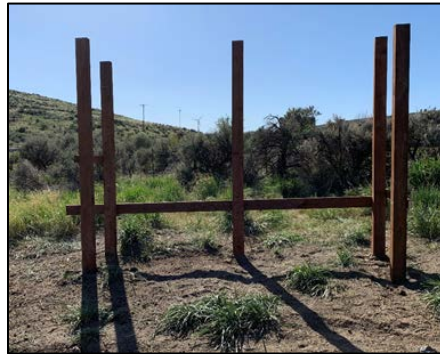
Support post set for volunteer kiosk construction project at the Corrals parking area
