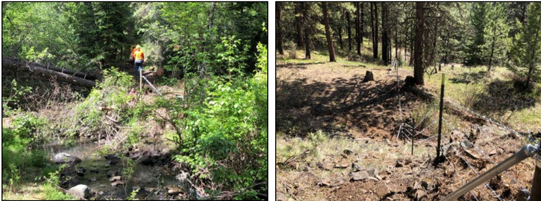
Line clearing and brace construction at Grouse Creek on the 4-O Ranch WLA, and some completed fence at the 4-O Ranch WLA
