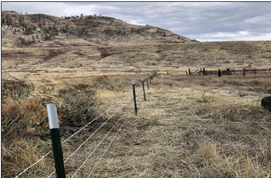
Staff member Medina, stretching wire and finished fence below Dunn Mountain – Photo by Dupont
