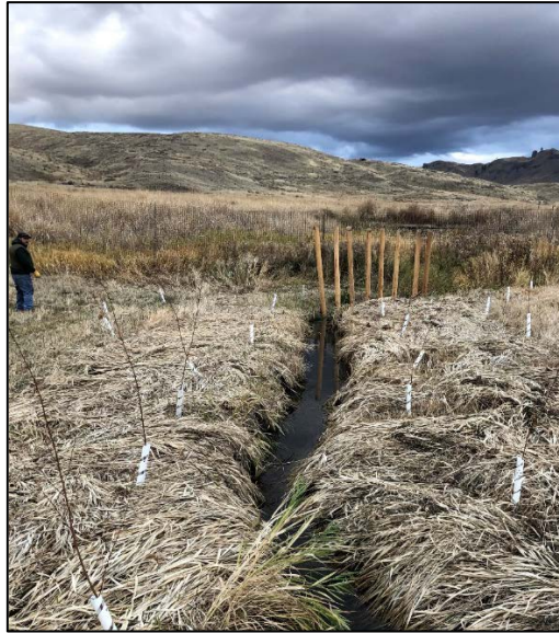
Staff member Medina checking out Beaver Dam Analog (BDA) #15, the last, farthest downstream BDA in the project area. BDA #15 was constructed in November 2021
