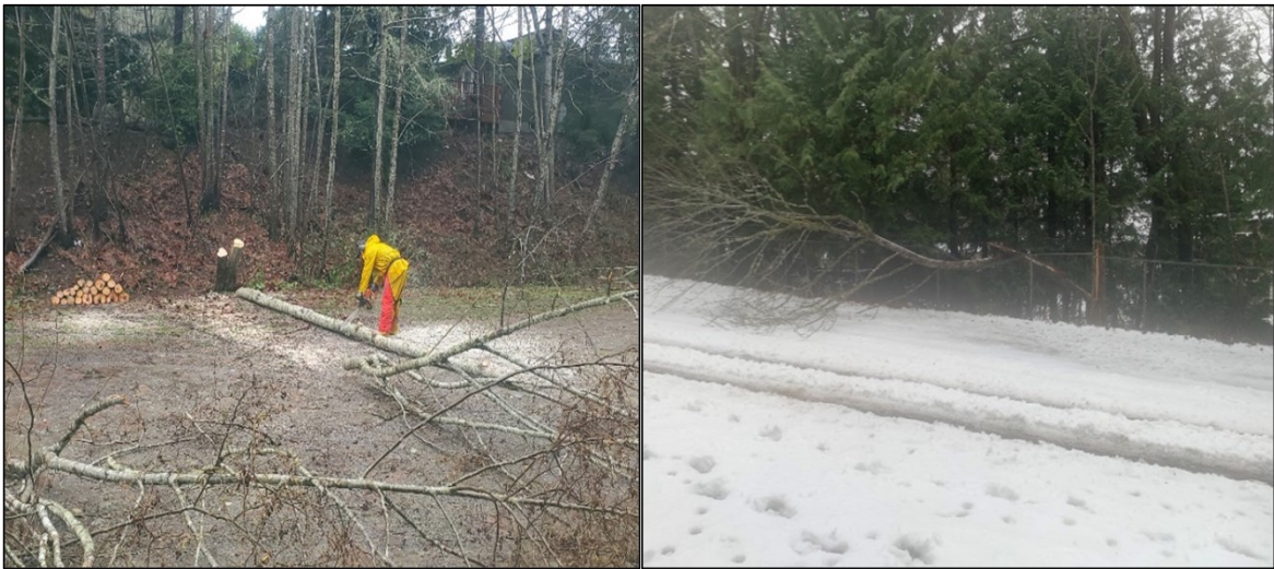
The access team members also removed downed trees from our recent snowfall and cleaned parking areas at Misery Point. Some minor fence repairs will need to be made
