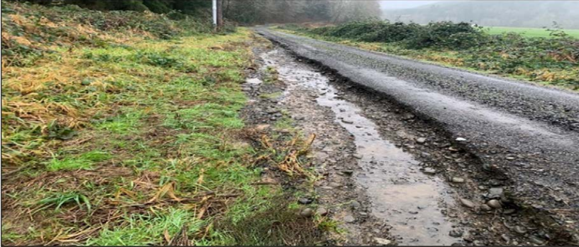
White Bridge- An excessive amount of runoff water caused damage to approximately 200 feet of the gravel road. Repairs will be scheduled in the weeks to come
