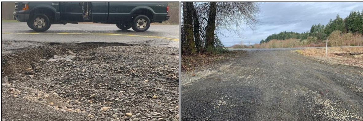
Flood water damaged the approach at the Porter Access Ramp. Excellent repair by team member Freimund
