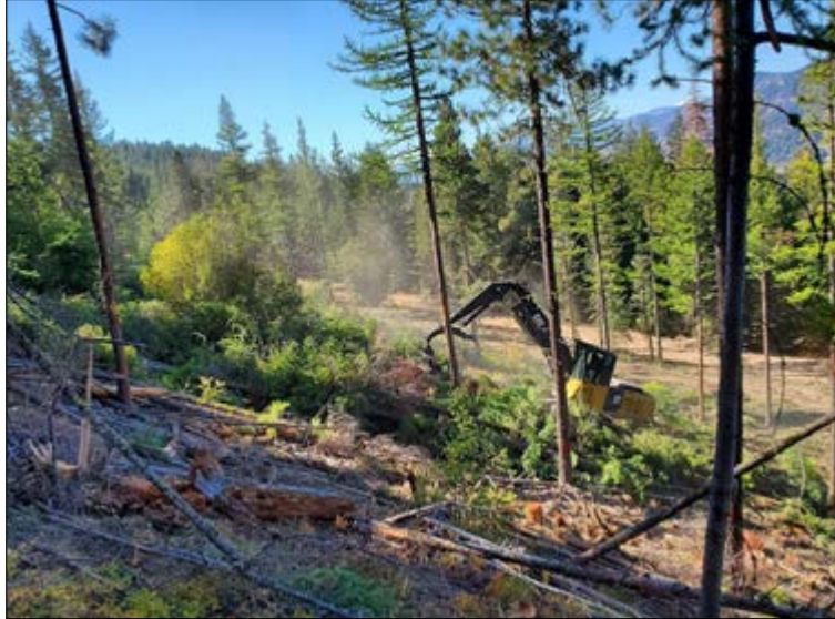
Loading machine “shoveling” cut trees in Unit 2 off a steep slope to a location where the wheeled skidder can relay the rest of the way to the landing
