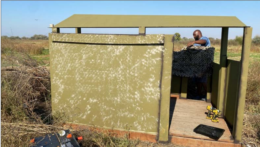
Volunteer Chris Oatis repainting the Johnson blind with a more subtle camouflage. Wildlife area staff will also be outfitting blinds with new grass mat coverings and camouflage netting
