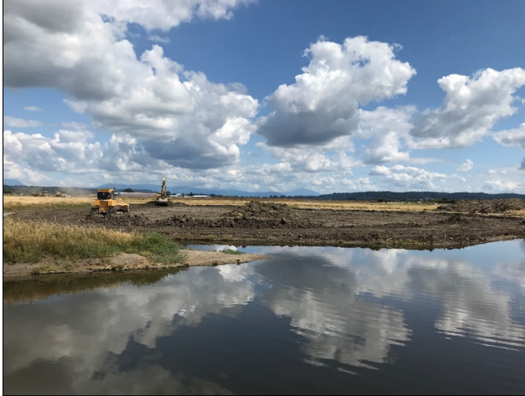
Equipment excavating tidal headwater areas that will be future intertidal habitat for fish and wildlife
