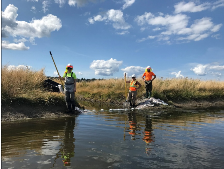
WDFW staff members removed fish from ditches before the contractor filled them in
