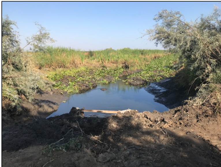
Brady Wetland outlet after removal of large mud beaver dam showing the top of a buried water control structure. Water level around six-feet lower than previously.
