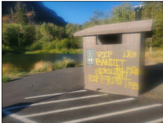
Graffiti damage at Tim's Pond
