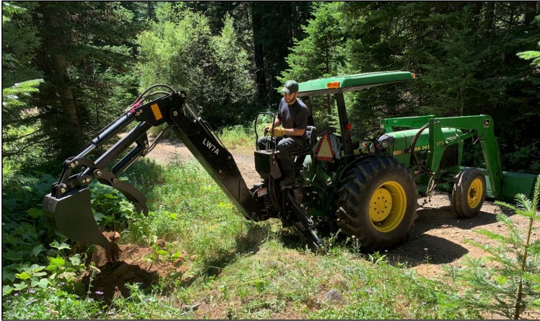
Blore digging holes for a new kiosk along the L.T. Murray's Walter Springs Road
