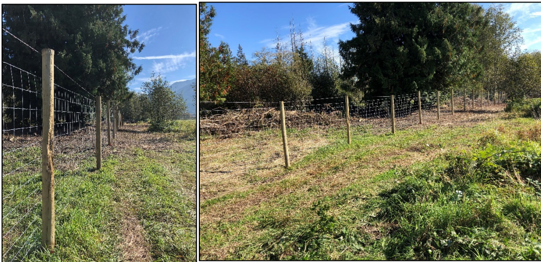
New elk exclusion fencing installed along a property boundary adjacent to State Route 20 in Skagit County
