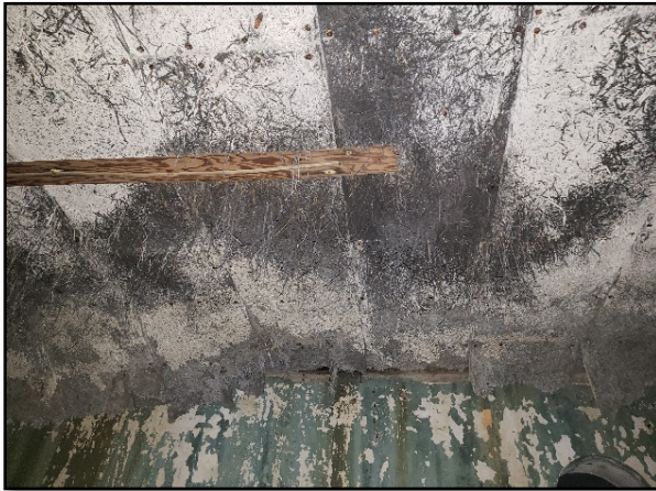
Ceiling area where bats roost
