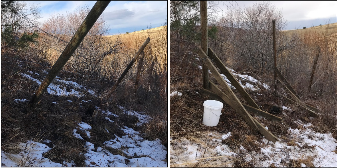
(Left) posts broke or rotted off at the ground and (right) braces built to stand posts back up
