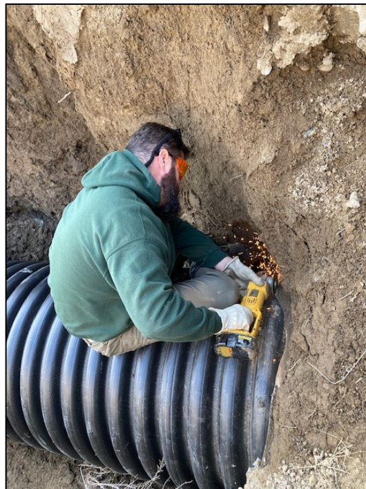
Ferguson cutting away metal from old culvert to facilitate installation of new pipe
