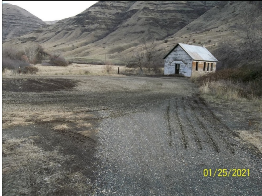
The old schoolhouse parking area on the Chief Joseph Wildlife Area getting a layer of gravel
