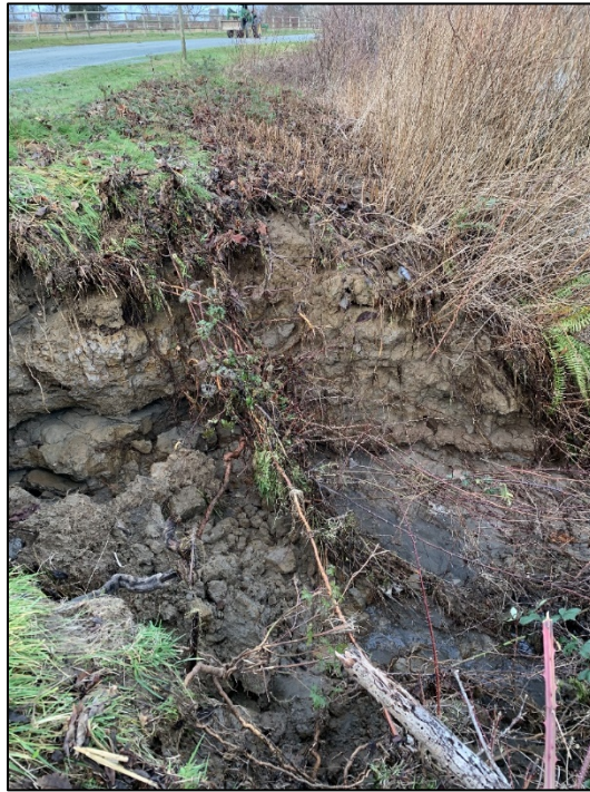
Recent storm damage on the Skagit Wildlife Area
