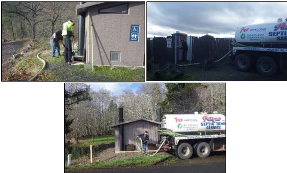
Vault pumping at Rowland Lake, Puget Island, and Onieda access sites
