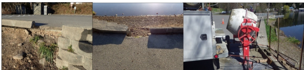
Broken curb at Mineral Lake
