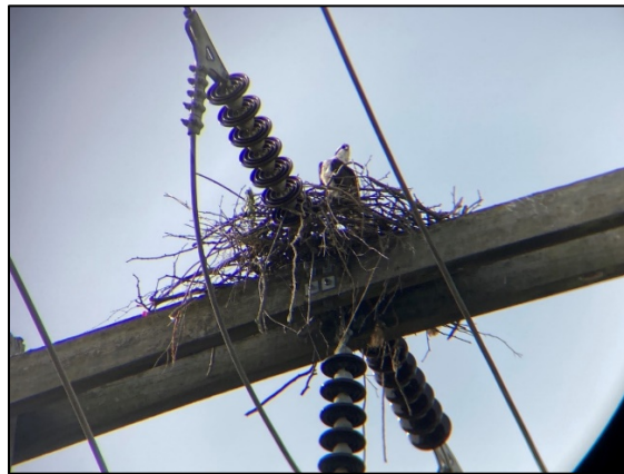
Osprey just starting to set-up a nest on energized powerline in Seattle. We like to keep electricity available and birds from any electrocution or fire situation! – Photo by Seattle City Light
