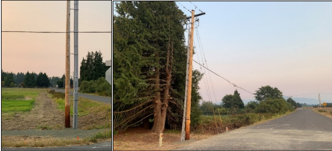
Left to right: New pole and covered trench with lines and wave cable is only line remaining to be removed
