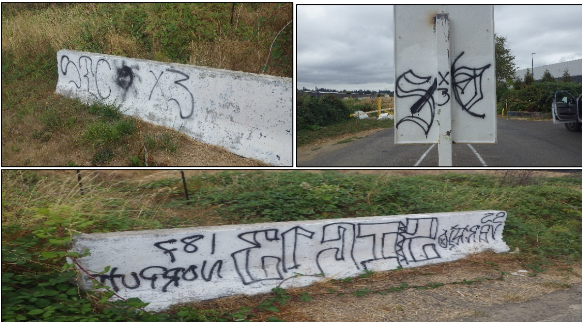
Continued vandalism at Vancouver Lake Access Site
