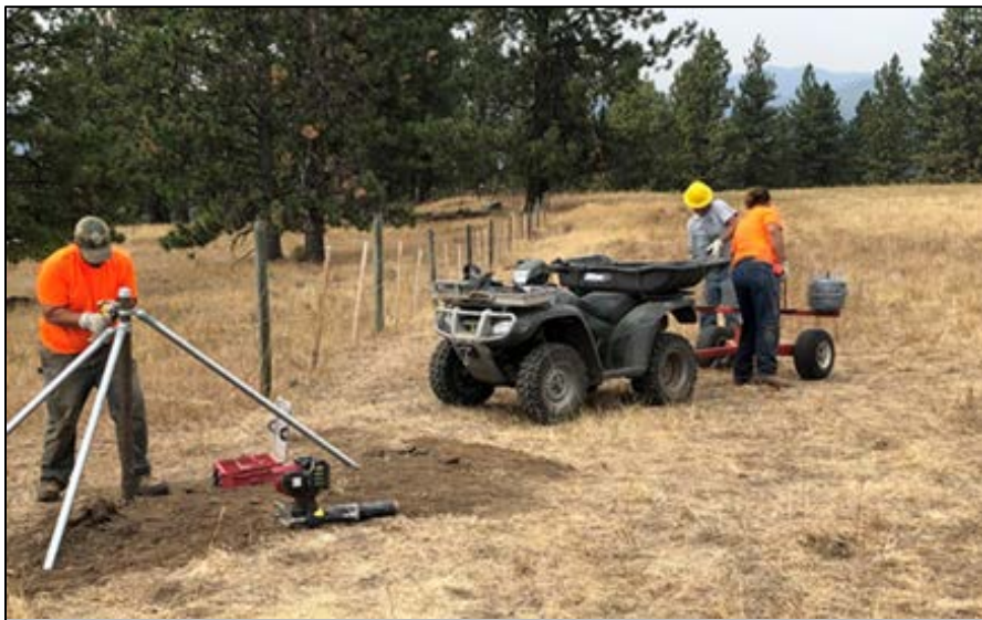
Blake Rimmelspacher, Scott McGee, and John Johnson preparing to attach wire to a new brace. The new fence intersects old fence at this location
