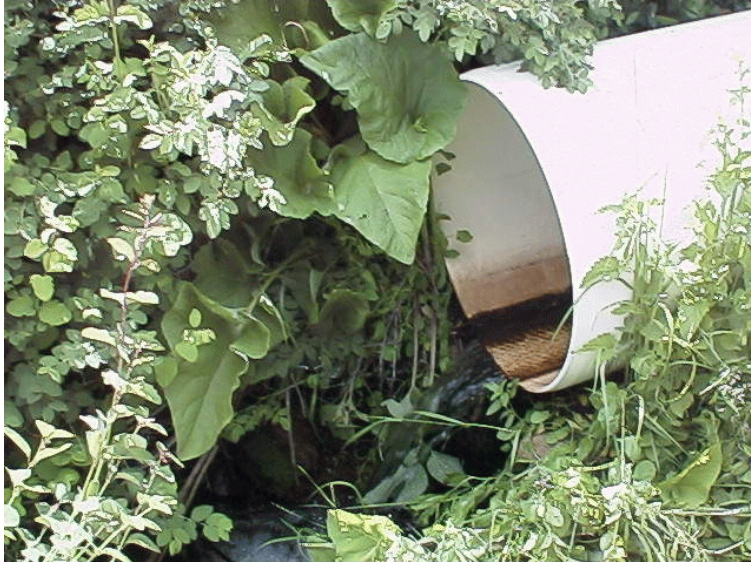
Photo 1. An unnamed tributary to the Twisp River. Although anadromous species are not present at this particular site, slope alone renders this pipe a total passage barrier for resident salmonids. The majority of flow percolates through the road fill.
