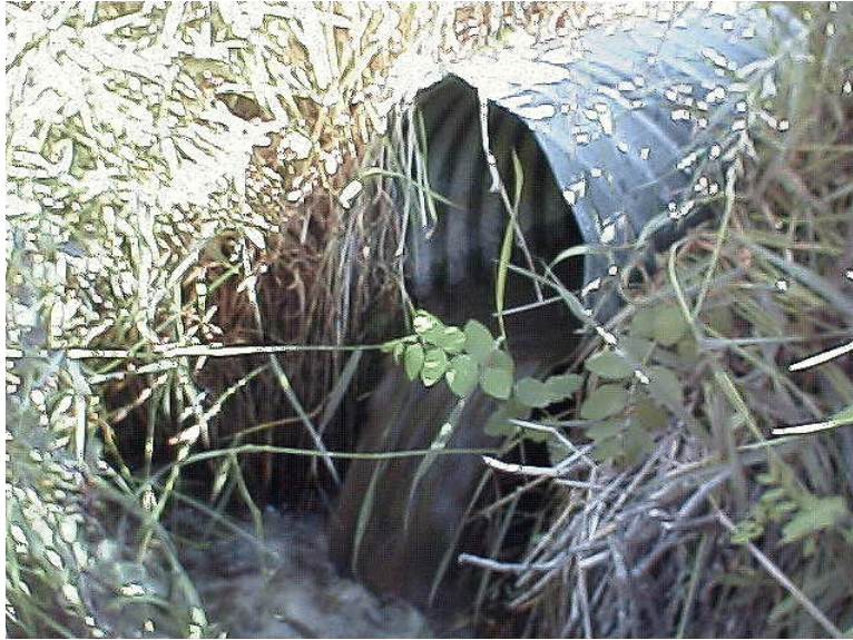
Photo 2. An unnamed tributary to the Methow River. Due to the inadequate size and slope of this culvert a large outfall drop has developed creating a near total fish passage barrier to resident fish. If the culvert was made passable, it is likely that anadromous species would utilize the habitat as well.
