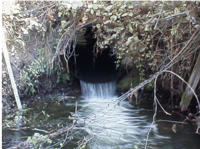
Photo 8. Bear Creek (48.0708). It is obvious, with this large of a plunge pool, that the culvert is undersized and was placed at an incorrect slope. This crossing alone renders 7,223 and 13,745 square meters inaccessible to several ESA listed salmonids.
