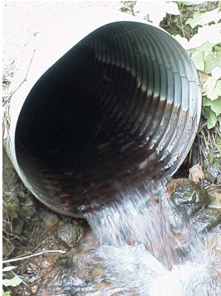
Photo 9. Bear Creek (48.0708). Due to the culvert being severely undersized and having a slope of approximately 7%, it has probably been a fish passage barrier since the time of installation. Notice the waterline on the inside of the culvert.
