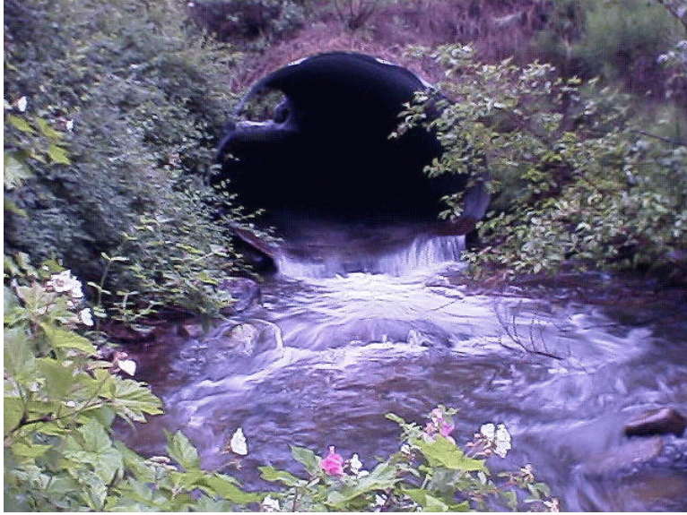
Photo 10. Cub Creek (48.0737). This culvert is the largest of all fish passage barriers on the Methow Wildlife Area. A slope greater than 1% and being undersized, designated the culvert a fish passage barrier. There is a series of large waterfalls several hundred meters downstream creating an anadromous barrier.
