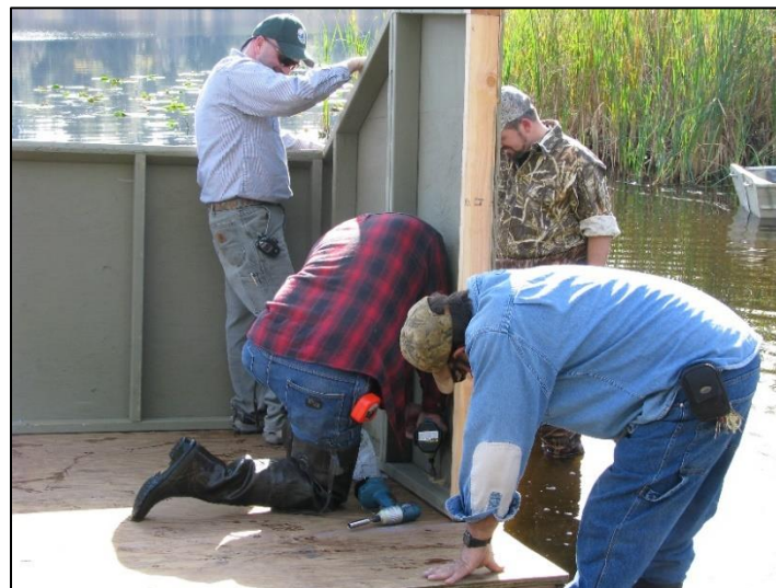
Members of the Washington Waterfowl Association assisting with construction of the Rapjohn Lake duck blinds, 2018.
